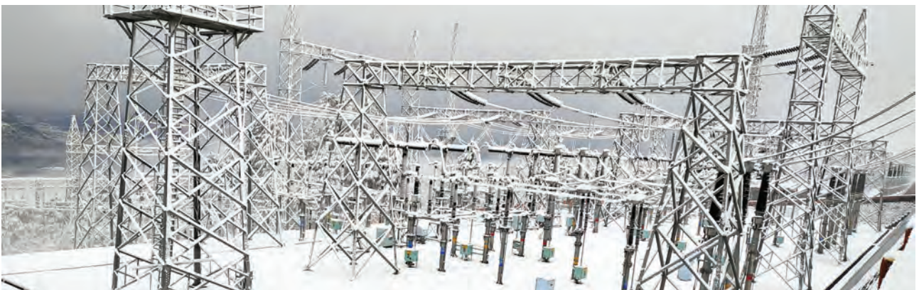
View of Pithoragarh Substation
